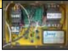
Electrical Junction Box
